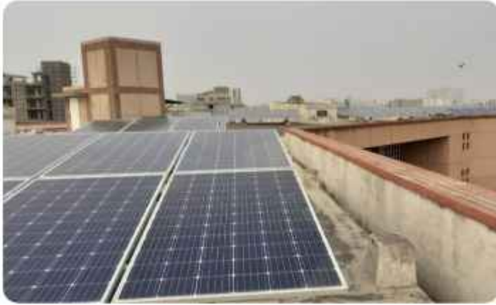
Solar Energy Plants (300 Kwp)
