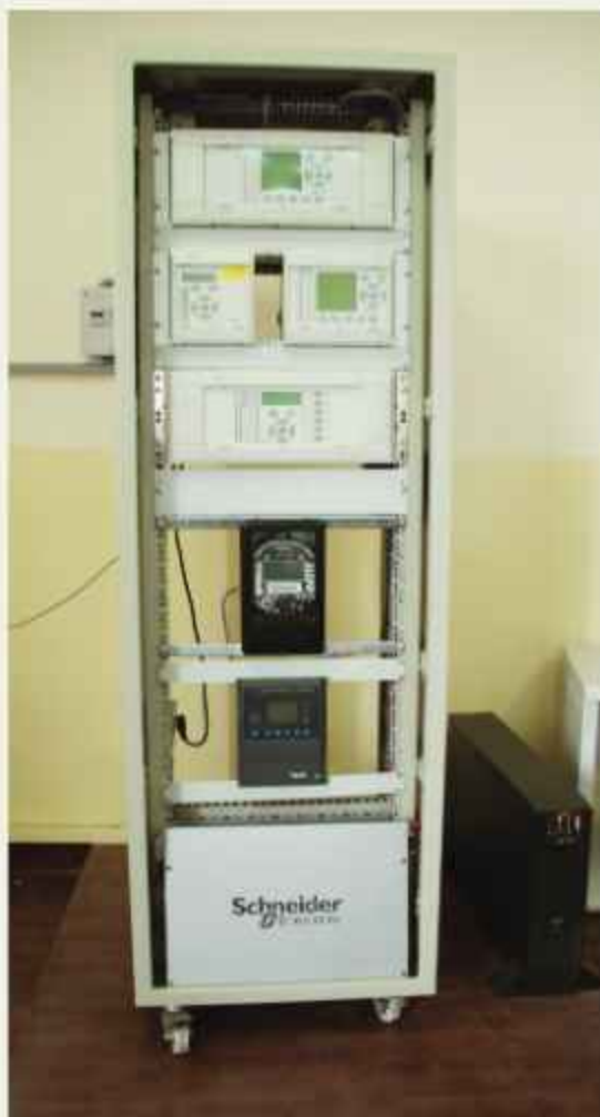
Substation Automation Panel
