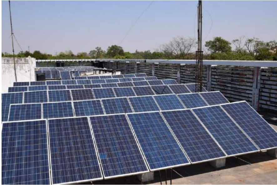
Fig. 46- Roof Top Solar Plant at CCL
