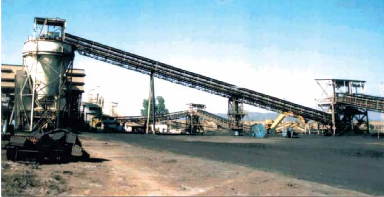
Sized Coal being transported through Conveyer Belt and stored in Coal Stacker to be washed in a Coal Washery
