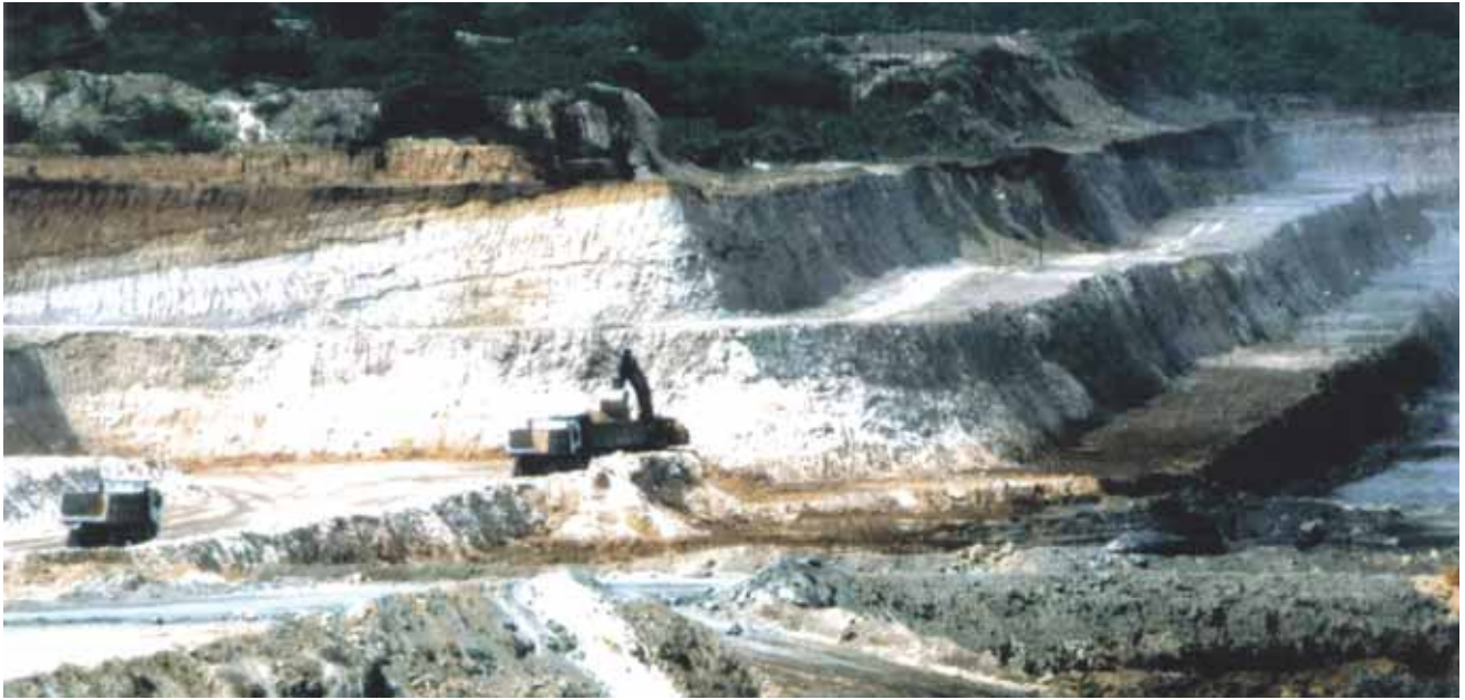
Over burden removal process in progress on bench of an Open-cast coal mine
