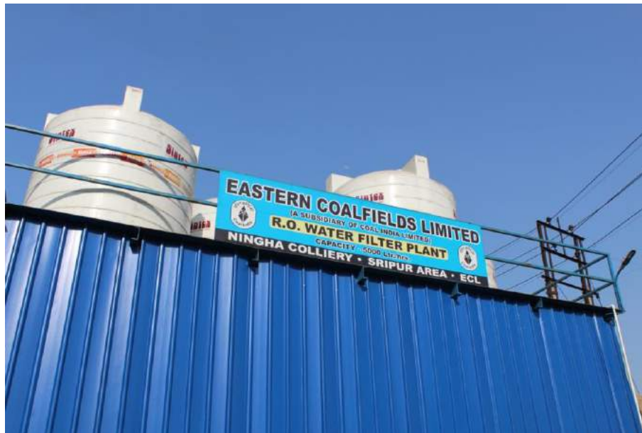
Fig. 36- R O Plant in ECL
