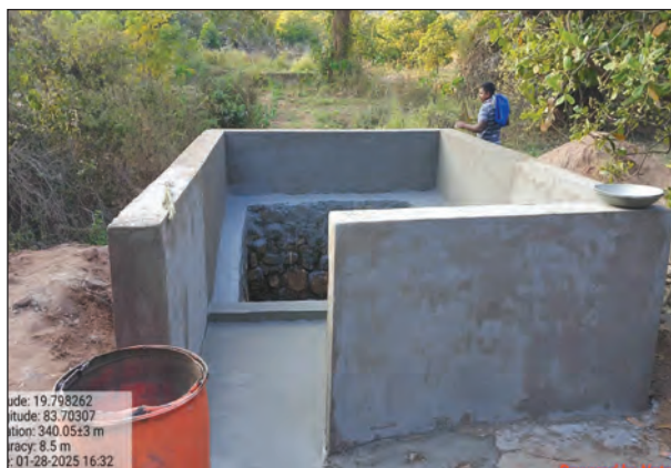
Barricading of open well
